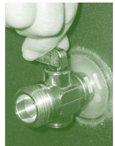
Close the drain valve
